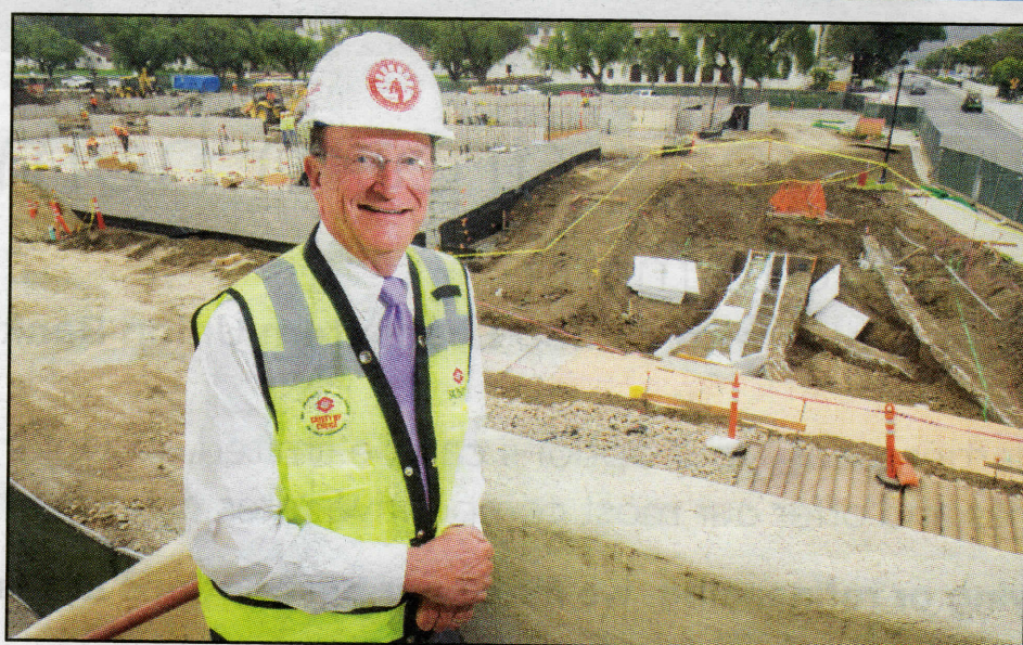
CSU Channel Island President Richard Rush stands near construction of a new chemistry lab building on the campus. CSUCI has embarked on a $600 million campus buildout.
