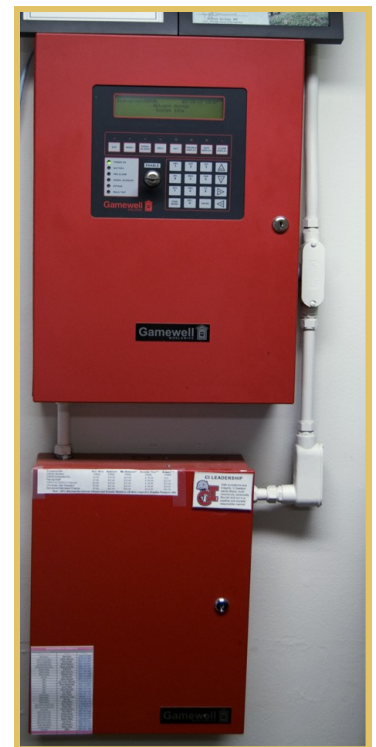
The Fire Alarm Control Panel in Arroyo Hall
